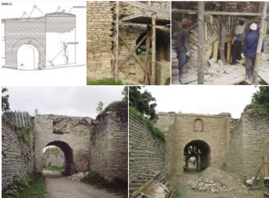
Upper Left: Architectural planning for restoration of Nikolsk Gate. Upper Middle: Restoration of a fort gate using authentic techniques and materials. Upper Right: Nikolsk Gate restoration work in progress. Bottom: (before and after) 2004 Progress: Conservation of Nikolsky Gate
