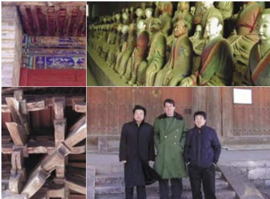
Upper Right: Damage from lack of maintenance and water leakage has destroyed over 30% of the walls, decoration and wooden sculptures of Foguang Temple.
