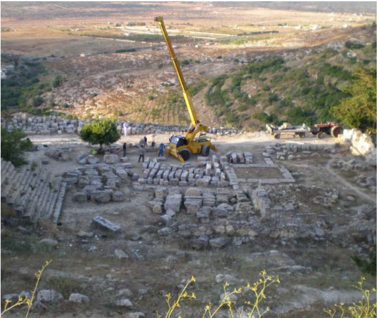
Cyrene, Libya: The amphitheatre of the Sanctuary of Apollo suffered damage from an earthquake in 4 th Century AD. Many seating stones in the cavea of this theatre have fallen and are displaced in a fragile condition to the Western end of the structure. In order to evaluate the need for consolidation of cracks in the rocks upon which the structure is built, stones must be carefully moved and registered. Anastylosis will be used to reconstruct that part of the Cavea damaged by the earthquake. Photograph: S Ensoli.
