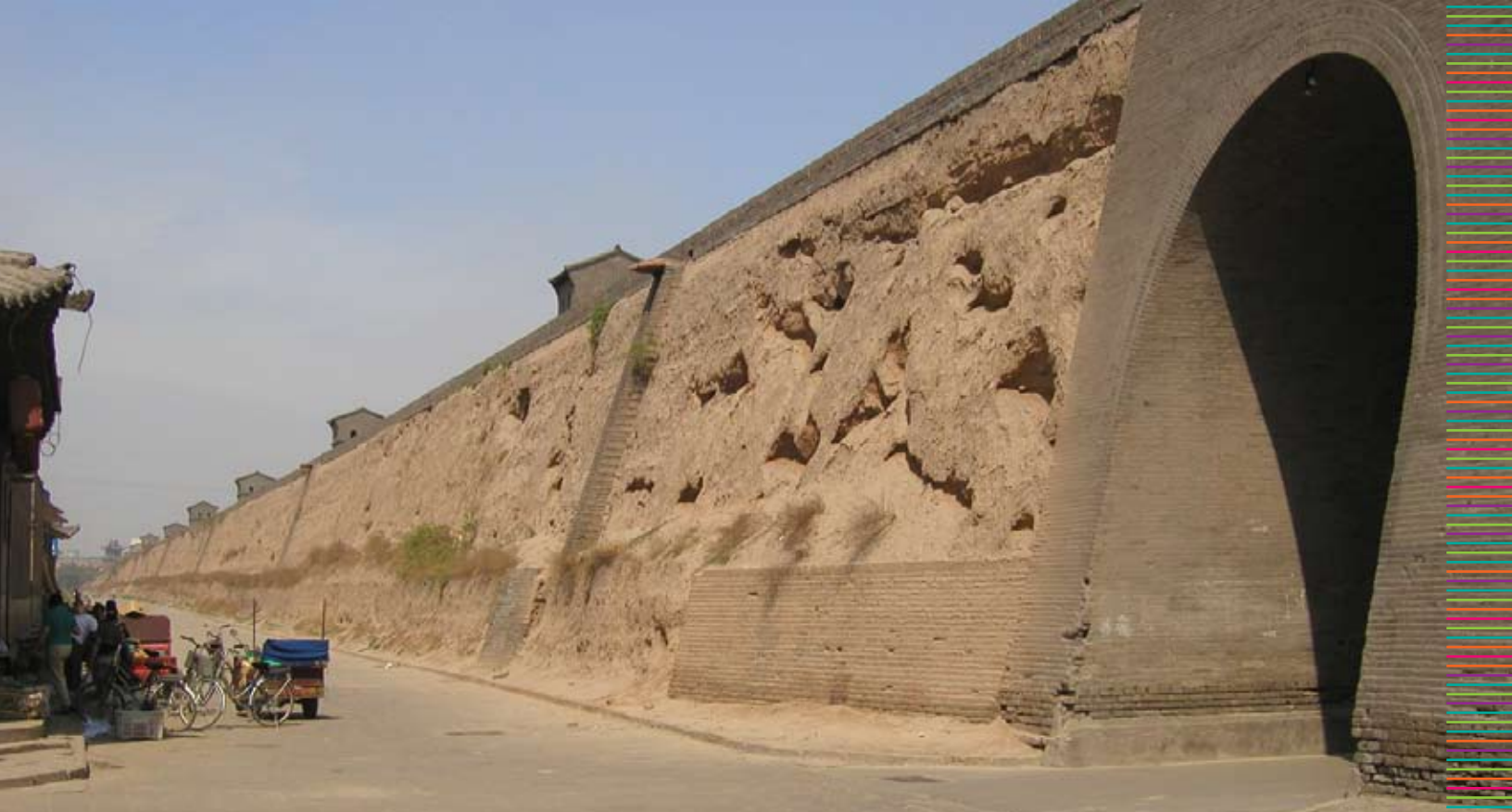
Pingyao Wall in need of restoration. Photo by Kuang-Han Li
