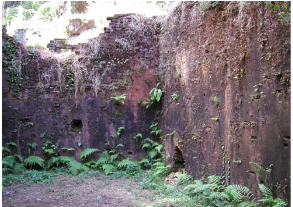
Vegetation overgrowth, one of the threats affecting various structures in the Sacred Temple Complex of Wat Phu, Laos. Photo by © Global Heritage Fund
