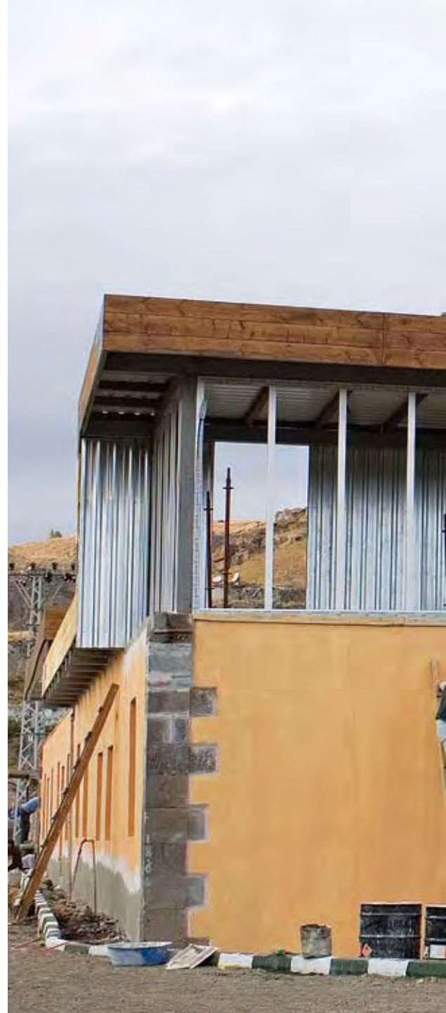
Restoration in progress on Namik Kemal Community Center, Kars, Turkey. Photographer: Yavuz Özkaya
