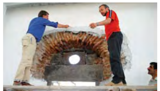
Plastering the Namik Kemal Community Center interior, Kars, Turkey. Photographer: Dan Thompson
