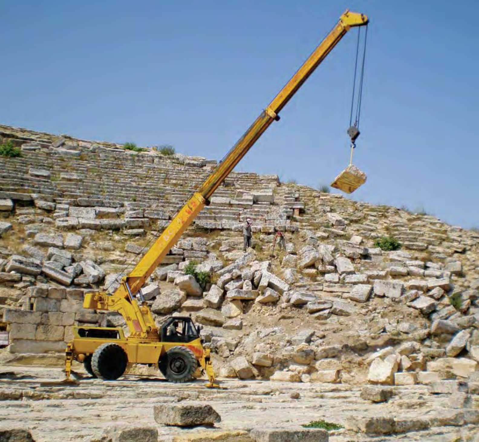
Using a mobile crane to stabilize and preserve the amphitheatre, Cyrene, Libya. Photographer: Serenella Ensoli
