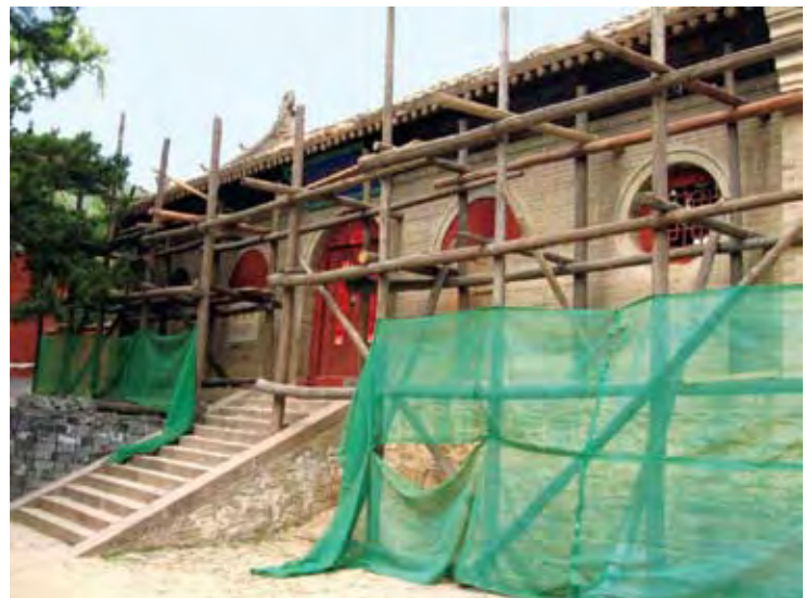
South facade of the entrance gate under restoration, Foguang, China. Photographer: GHF
